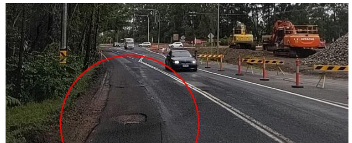
Image: The ADL system identified a pothole defect on the road.
